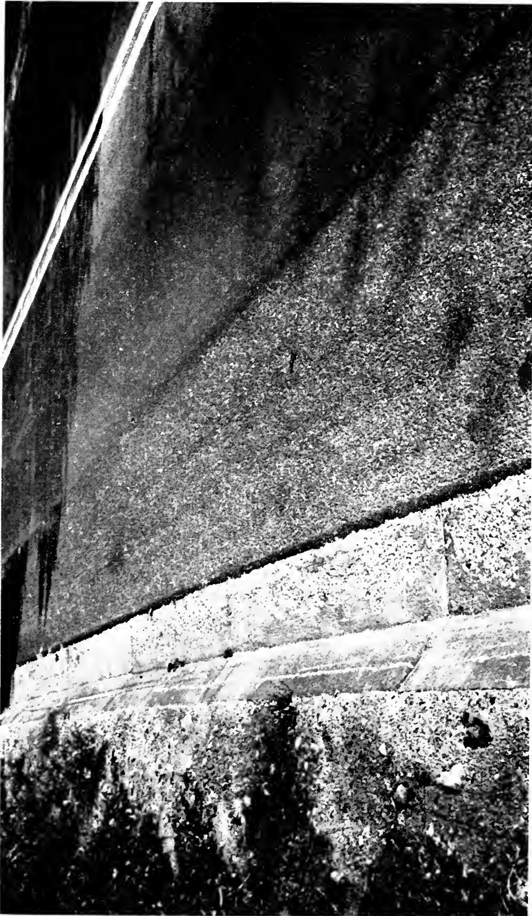
GOOD EXAMPLE OF PROPER INSTALLATION OF CONCRETE REBUT AND CUTTER WITH BITUMINOUS TREATED SHOULDER. STABILIZED TO PREVENT EROSION
